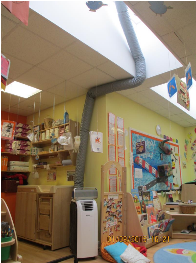
Image 5 – Cooling units currently used inside the nursery.
